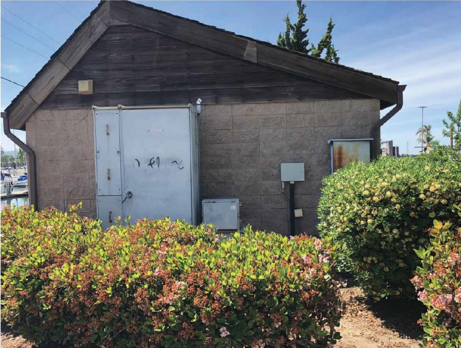
PHOTO OF UTILITY BOX GROUPING ON WALL
